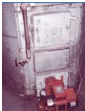
The owner of this 1916 furnace, which had been converted from coal to oil, recently replaced it with a high-efficiency oil furnace.
